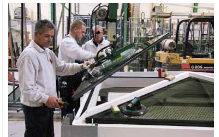
THE CUPOLAS ARE GLAZED WITH TRIANGULAR GLASS PANELS MADE BY SCHEUTEN GLAS IN HOORN.
