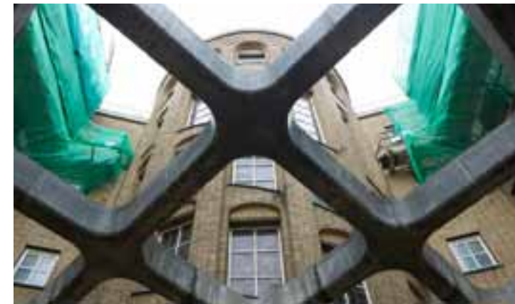
NARROW SEAMS IN THE CONCRETE BETRAY WHERE THE FORMWORK ELEMENTS WERE ATTACHED TO EACH OTHER. THEY WILL BE FINISHED INVISIBLY AT A LATER STAGE.
